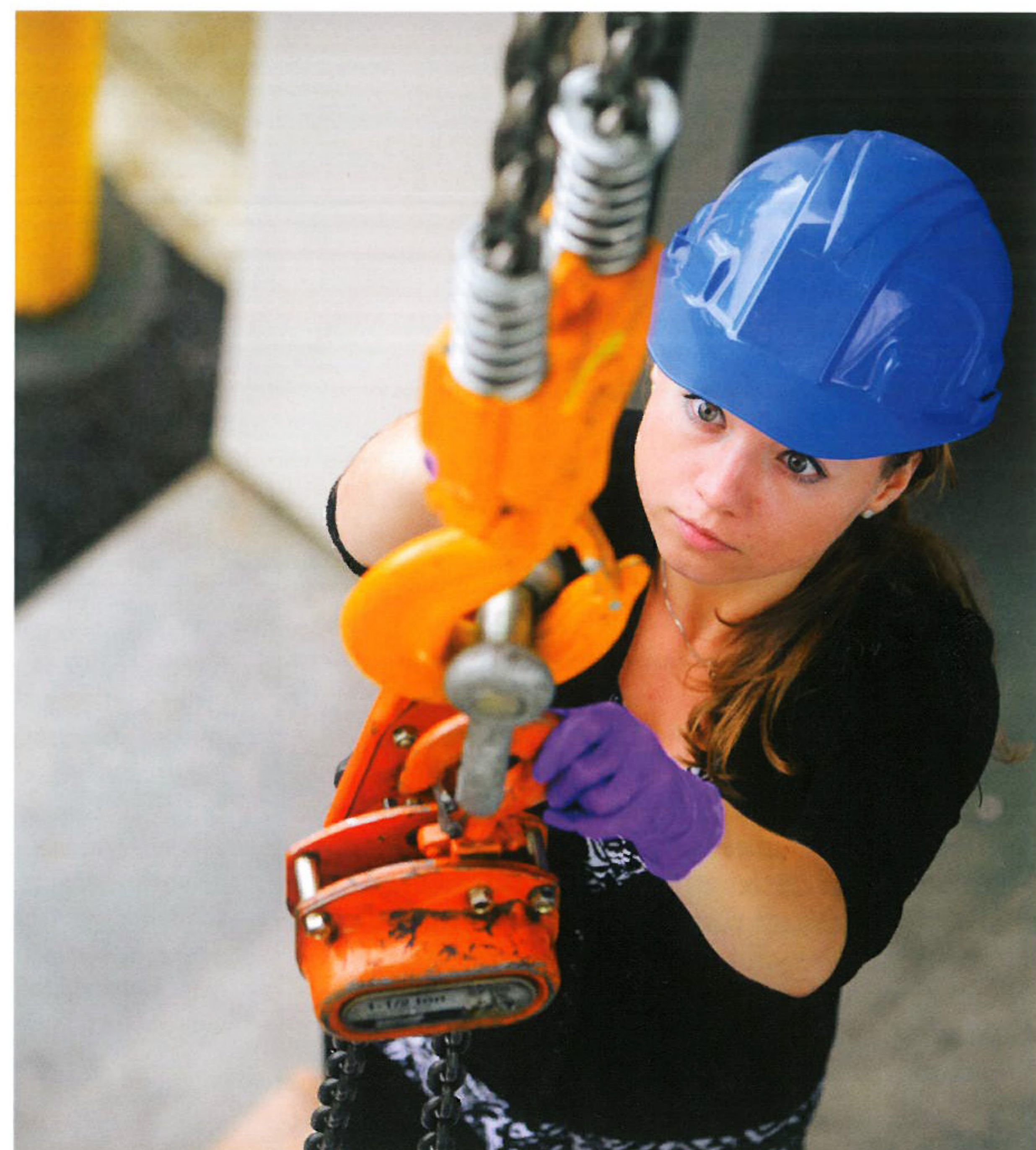
Izabela Gutowska attaches a ceramic block to a crane during core installation. (Photo: Karl Maasdam)
